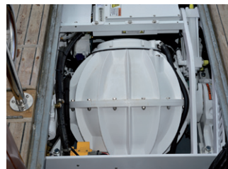
Here the gyro is preceding aft, thereby countering roll to the port side.
