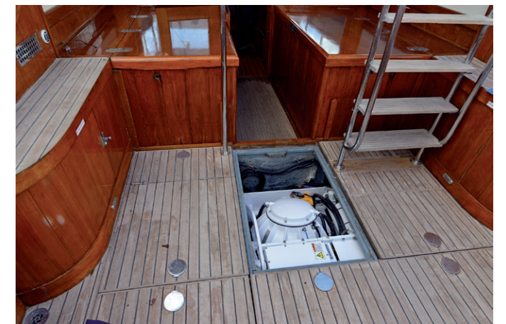
In real terms, Seakeeper 5 is a compact system even for this 36ft Hagg and fits quite easily under the cockpit.
