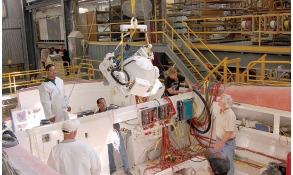
A Seakeeper gyro stabilizer goes into a new 55-foot Viking at the builder's New Gretna, NJ facility.
