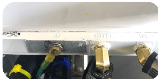
Motor drive ground connection
