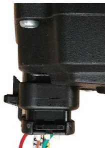
Seakeeper 1 Curtis drive connector securely fastened.
