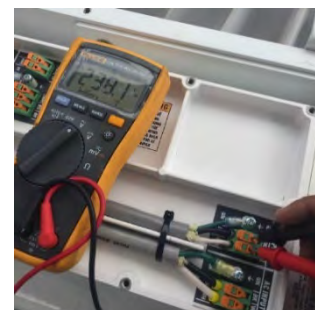
Testing SW Pump voltage
