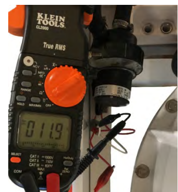
Image of technician back probing glycol pump connector for voltage
