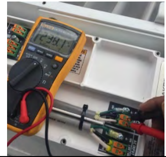
Testing SW Pump voltage
