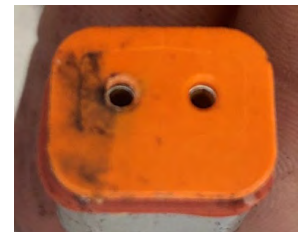
Evidence of moisture intrusion in a harness connector
