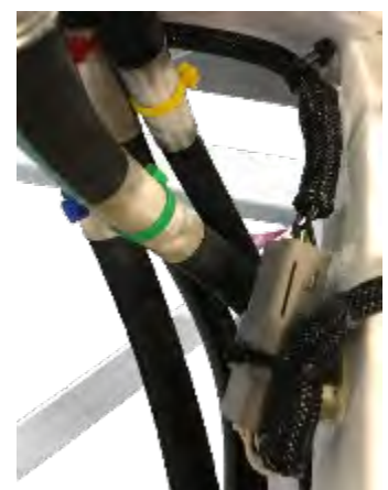
Photo showing location of Guide Band connector inside foundation near guide band bracket and below manifold.
