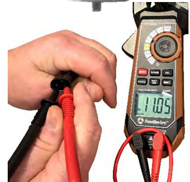
Meter in this photo is displaying 11.05 KΩ.
