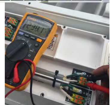
Testing SW Pump voltage
