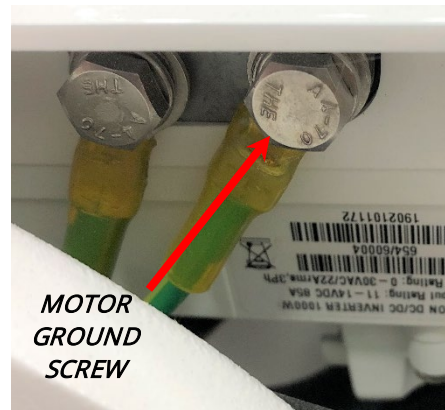
Figure 13: DC motor ground cable
