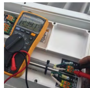
Testing SW Pump voltage
